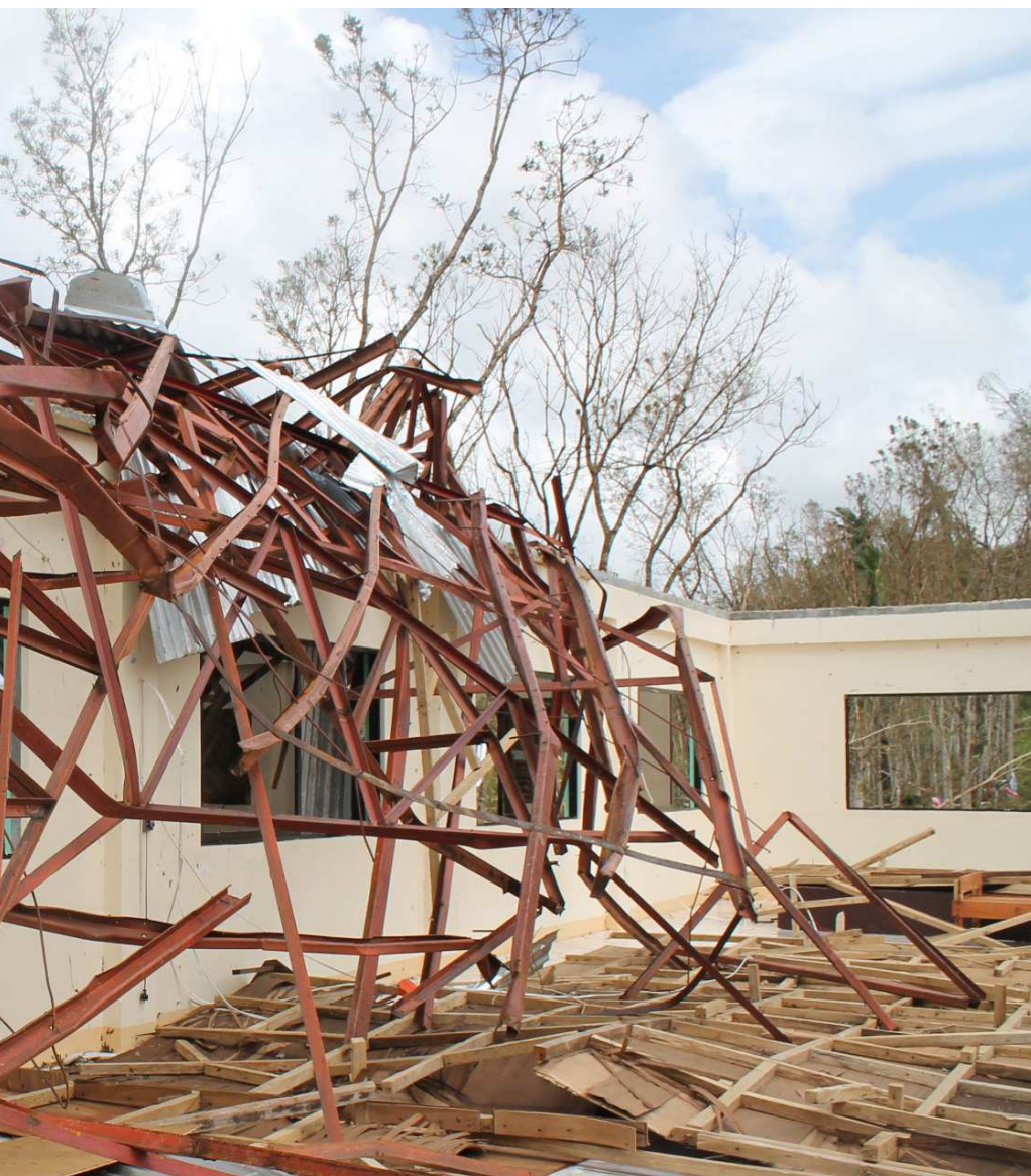
viewing of the damage caused by the Typhoon Yolanda.
