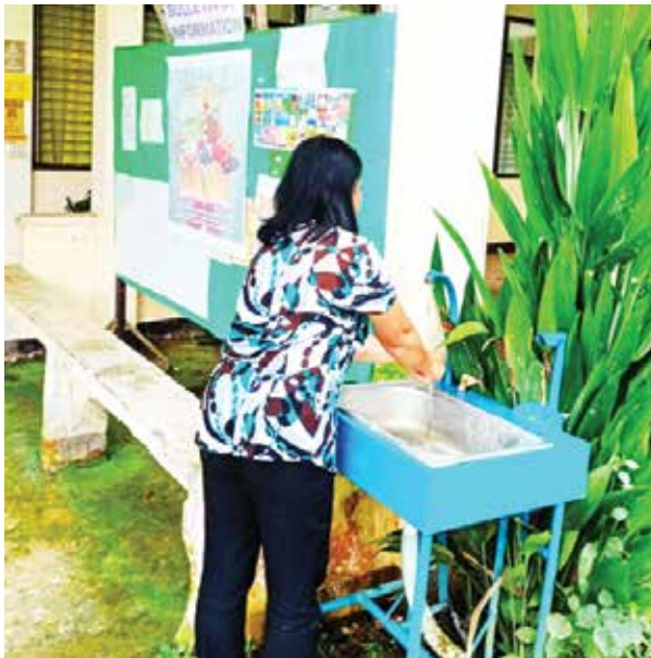
■ Acquisition of handwashing facilities
