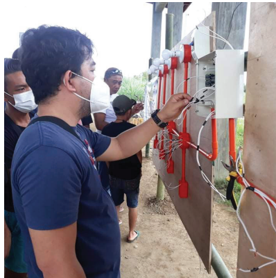
Skills Training on Building Wiring Installation Trainer: Engr. Ronnel P. Babis Brgy. Cogon, Panitan, Capiz last February 19-March 6, 2022
