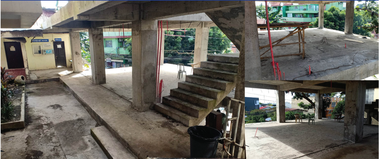
COMPLETED PHASE 1 OF THE EXPANSION OF THE GABALDON BUILDING ANNEX 3 (STRUCTURAL (COLUMNS, SLABS AND STAIRS) FOR A 3-STOREY BUILDING)
