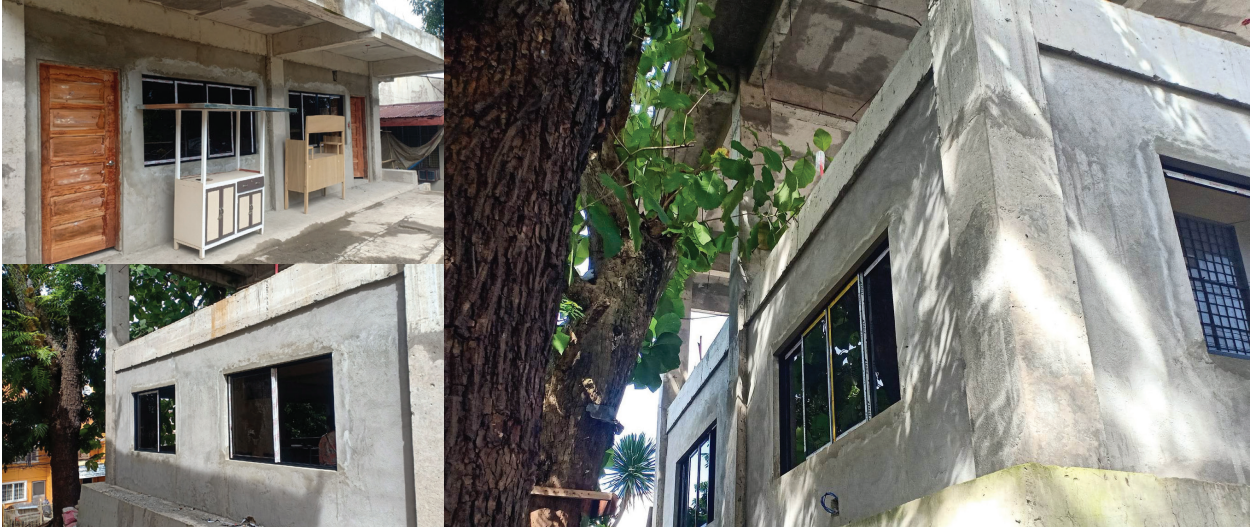
COMPLETED PHASE 1 OF THE EXPANSION OF THE GABALDON BUILDING ANNEX 2 (A 2-STOREY BUILDING WITH THE WALL, WINDOWS, AND ELECTRICAL WORKS ON THE GROUND FLOOR)
